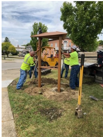
Message Board installed On Market
